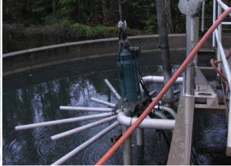
Shown with guiderails, retrieval system, and partial rubber hoses
